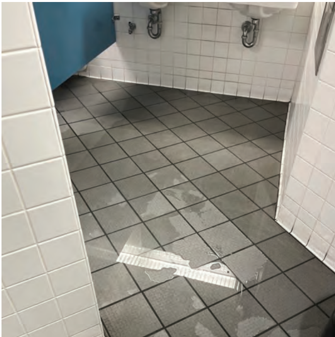
The women's bathroom (next to the men's that flooded yesterday) is starting to flood out of the floor drain.
