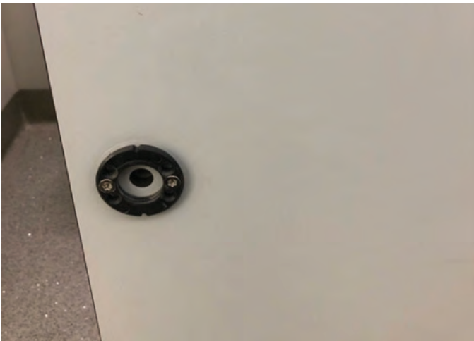
The woman's restroom by United level six the door lock broken.
