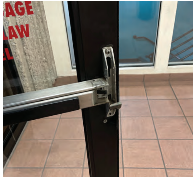
Door bar on northwest corner of parking garage level 7 elevator lobby is broken.
