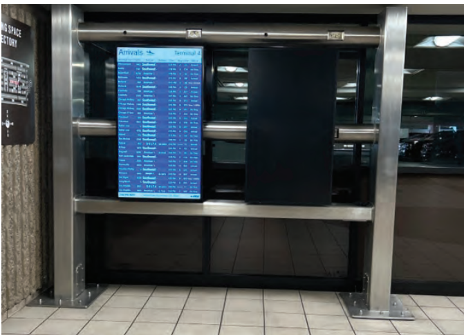
West end parking garage lobby – one of the flight boards is out.
