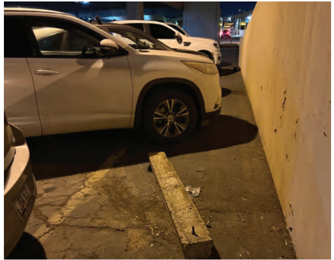
North Economy garage lower on the end of the row D-2, there are two tire stops with rebar sticking up against the wall by the down ramp parking spaces.
