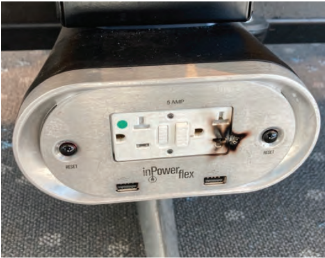
Gate E12 seating area. Broken off prong in outlet. Passenger was shocked.
