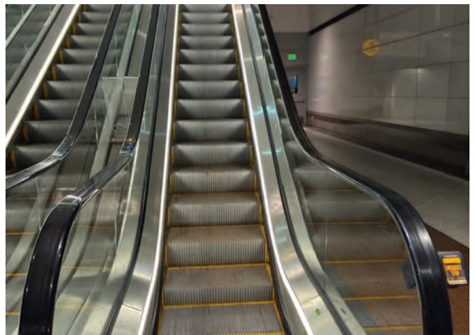
Escalator outside train C concourse south side is broken below McDonald's.
