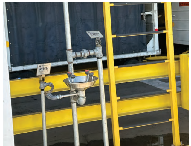
Eye wash station in front of United bag room not working, shower does not function, water is brown. This is a safety concern.
